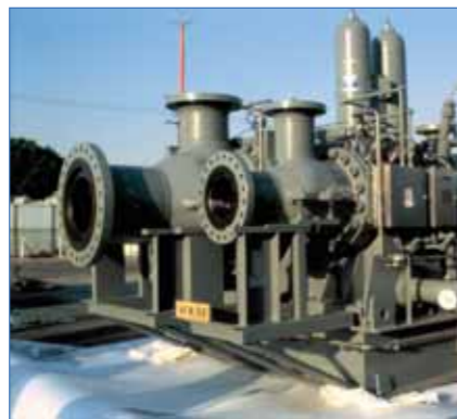
A three stage expander mounted on a single integral gear. This natural gas pressure letdown application handles 68 MMSCFD (76,000 Nm 3 /hr) and produces 5-MW of electrical power.
