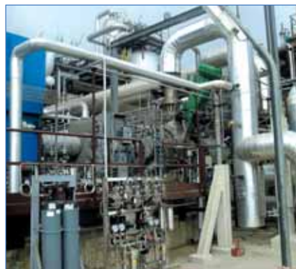
Located in Sicily, Italy, an Integrated Gasification Combined Cycle facility uses a GE Turboexpander-Generator to reduce the fuel gas pressure into its gas turbines. At the same time it produces 10-MW of electricity by expanding 313 MMSCFD (350,000 Nm 3 /hr).
