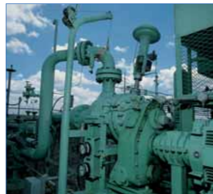
A pressure letdown installation recovers 1,000,000 kWh/yr from a southern California, US municipal natural gas pipeline.
